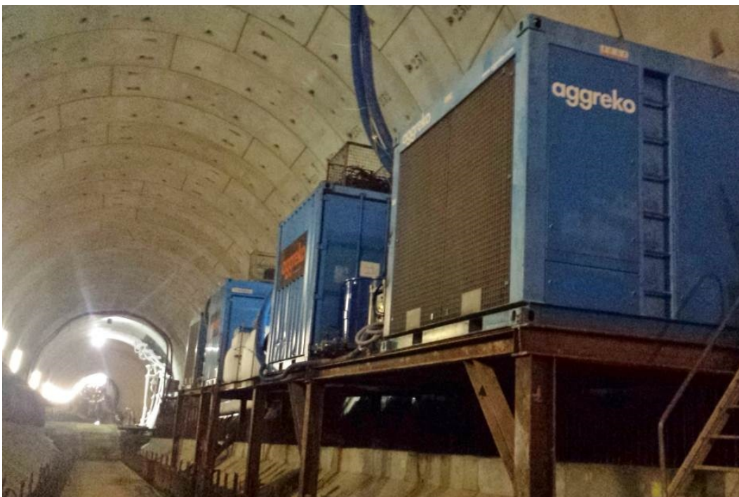
Two freezing units inside the main tunnel
